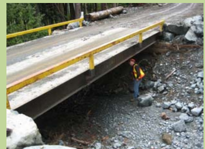
The field audit included a review of recently installed watercourse crossing structures to verify the protection and maintenance of water resources.
